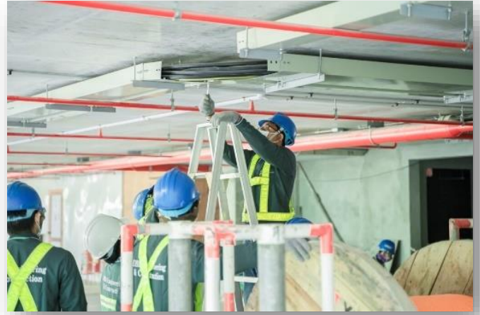
Mechanical and Electrical
